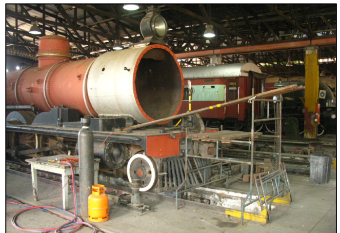
P04 - Class 6A 473 'Charlotte' with the first few boiler tubes having been withdrawn. The other tubes had already been split and crushed at the front end.
