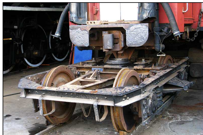
P02 - The multistage process of rolling the bogie under the coach again, complicated by limited jacking heights.
