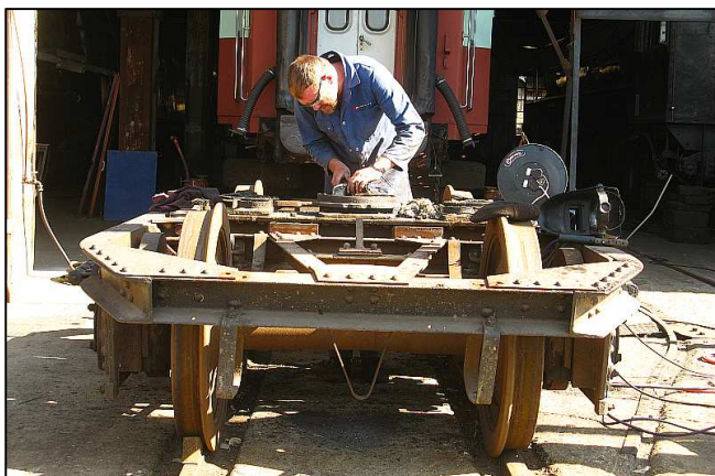
P01 - Grinding the new welds on the cup-shaped boss for the Locomotion Coach’s bolster pivot.
