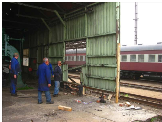
P06 - Some jacking, bracing and repair work taking place on the old forge building. One loose panel was completely removed so the building is now shorter. This isn't part of the original 1885 work, but those timbers are old enough!
