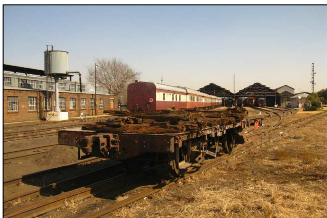
P03 - Some of the rotted wooden sleepers removed from the old staging yard and replaced with concrete sleepers.
